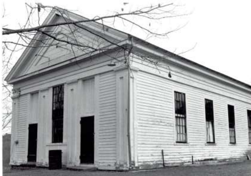
The Hall pictured c. April 1995 prior to renovations. Lots of rot along the south side ground, lots of busted windows, no pavement up to both doors, no railings, slate roof needed repairs. The memory garden had not yet been planted. You should have seen the damage and repairs needed inside!
